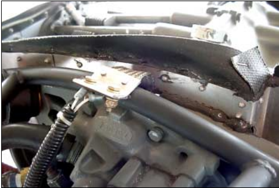
Center rear baffle (installed).
