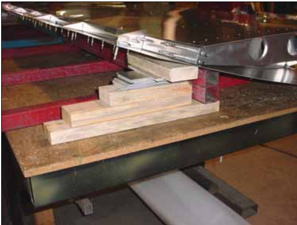
Extra spacer blocks under the inboard end of the rear channel to level the top of the channel.
