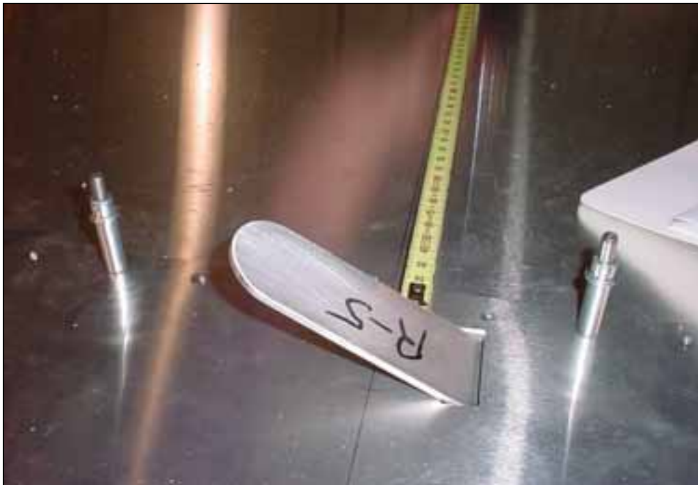
LAYOUT: From the aft edge of the strut fitting, layout 355mm to mark the aft end of the angle 7V8-4SP
