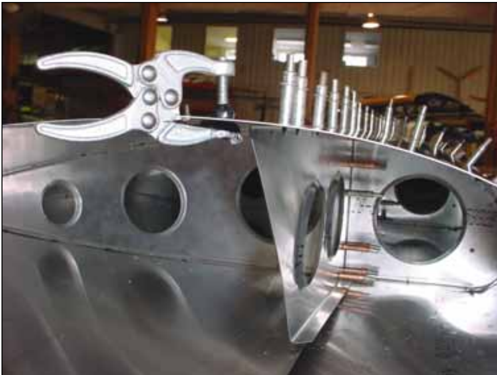
Check: edge distance of the rivet line in the top flange of the spar tip.
