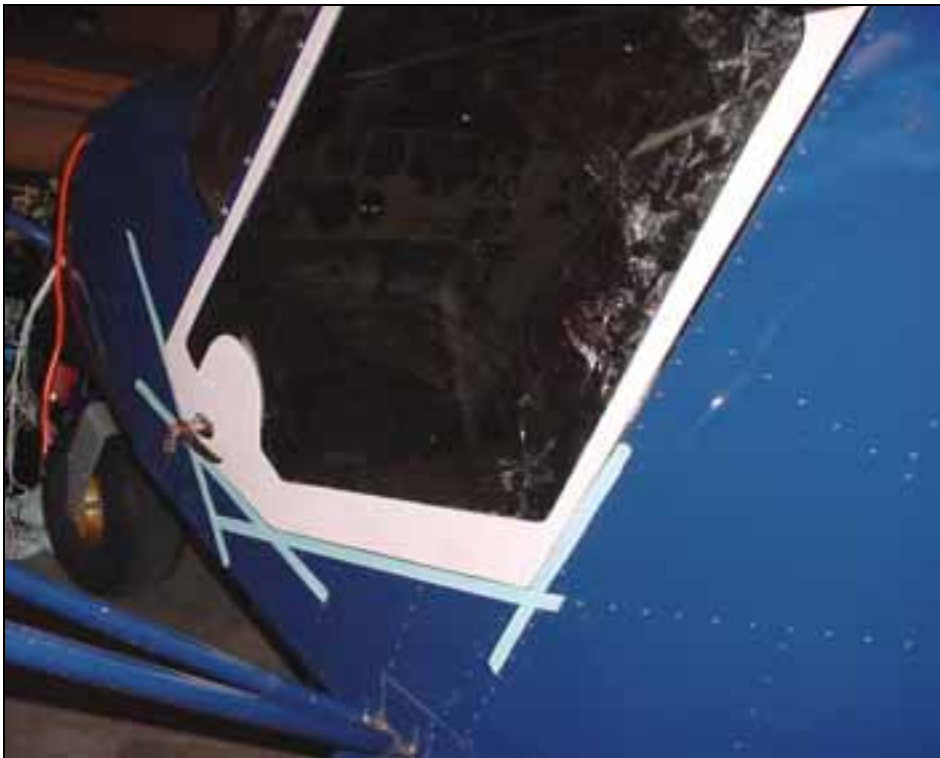
Trim the bottom edge of the door even with the top of the tape line.
