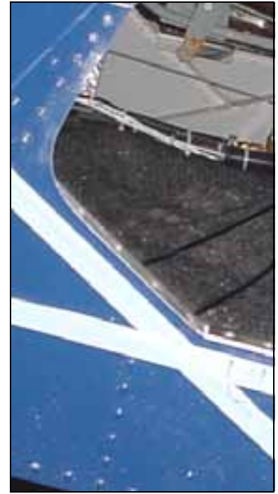
Top edge of the tape is approximately 6mm from the door opening.
