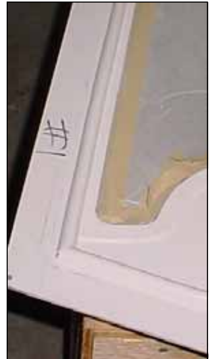
Fiberglass door supplied with a sharp point in bottom front corner.
