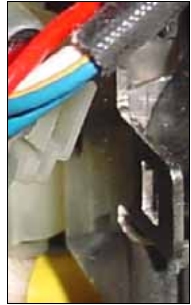
Square hole in steel mounting bracket.
