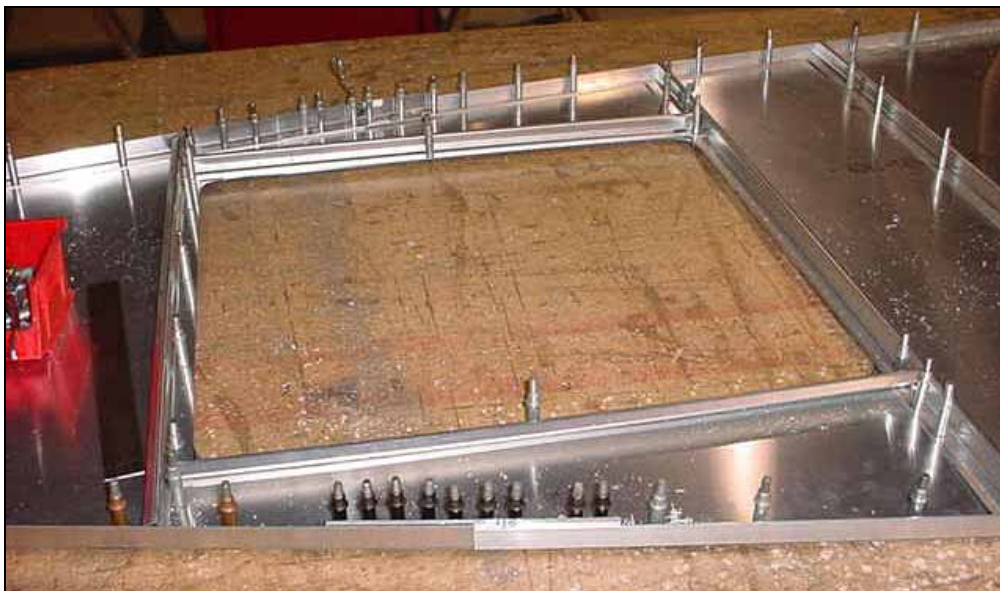
Cutout in fuselage bottom skin is reinforced with Z angles all around.
