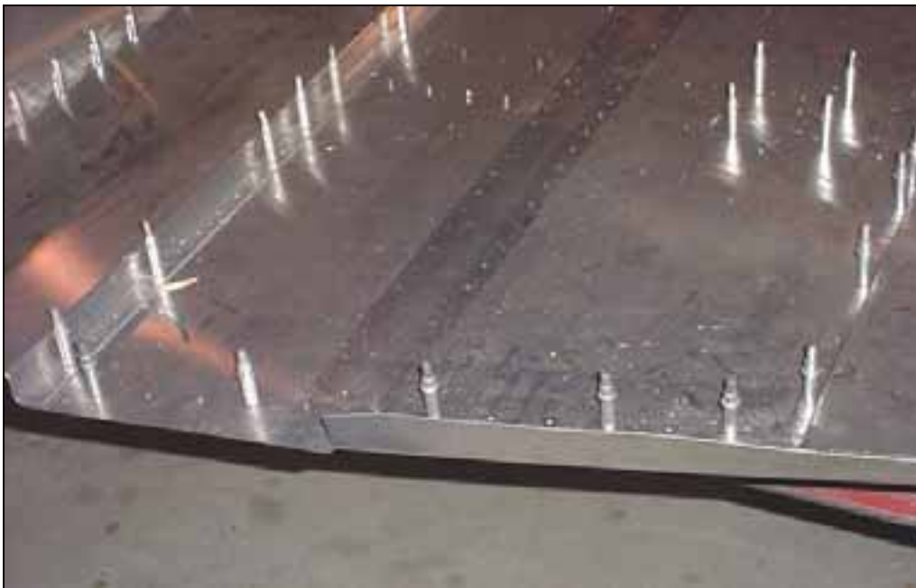
Side flange on the cabin floor skin 6B10-1 (area in front of spar).
