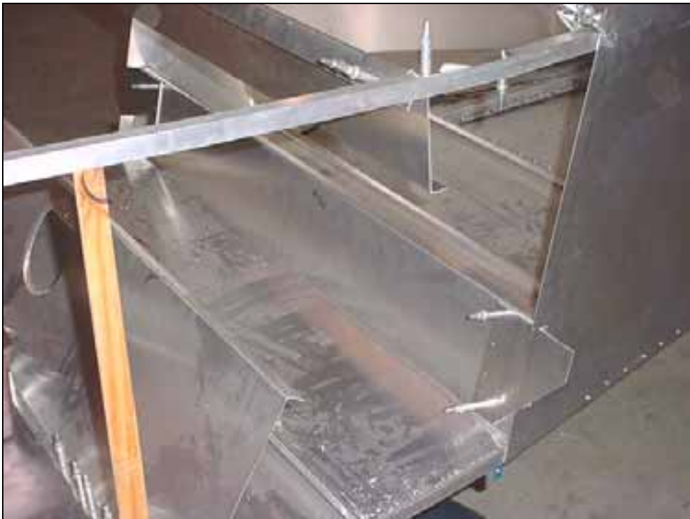
Rear fuselage with rear frame channel 6B5-2 installed. Photo looking towards the rear.
