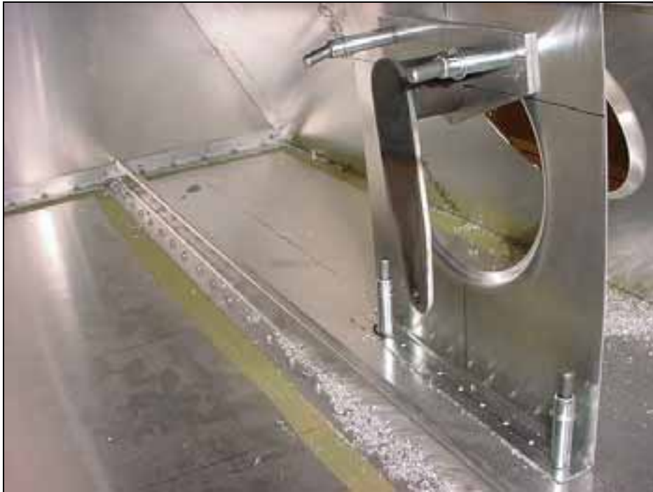
Rear view looking forwards. Drill and cleco the bottom flange of the rear torque tube bearing support 6B17-1 to the bottom skin 6B1-4
