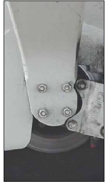
Above photo shows gear installed opposite of recommended direction.
