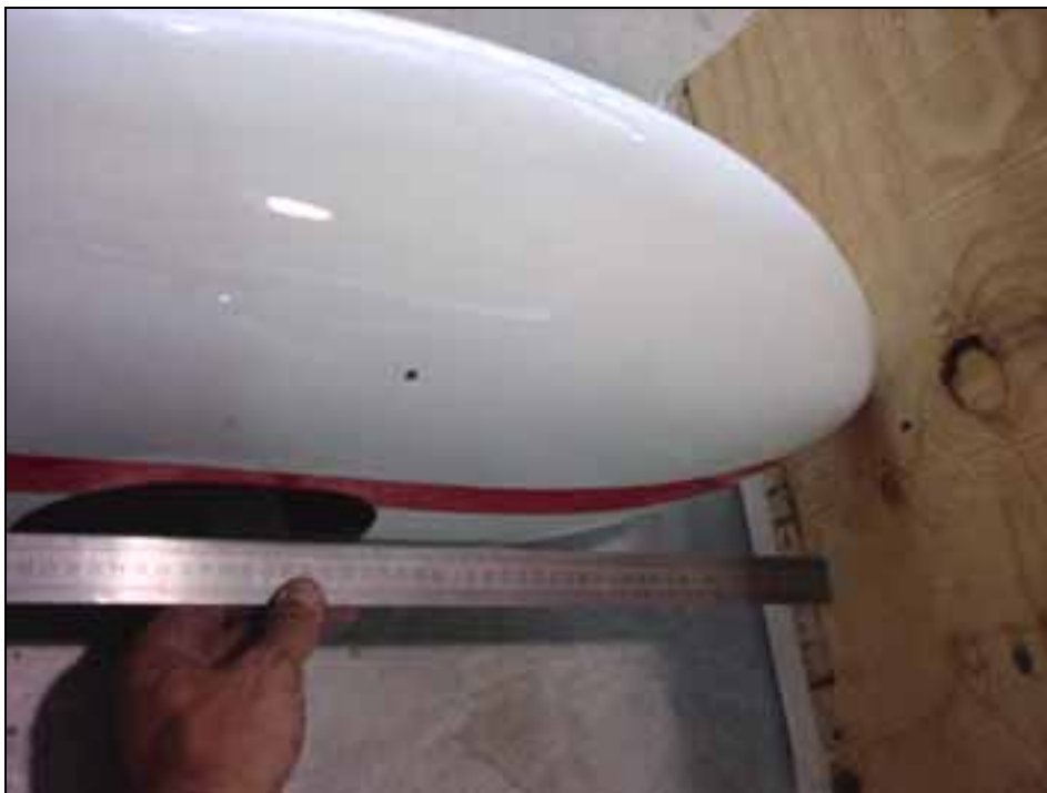
Layout the front and rear edge of the cutout for the gear and calipers.
